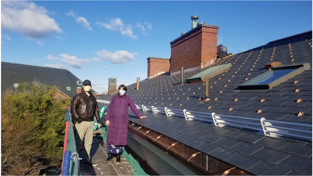
This is a new slate roof and copper gutters that my guys installed at the Kennedy Center, 23 Moulton St., Charlestown, MA. The job started late Aug 2020 and was done by the first week in November. Pictured are architect Shawn Willett (left) and KFC executive director Thara Fuller.
